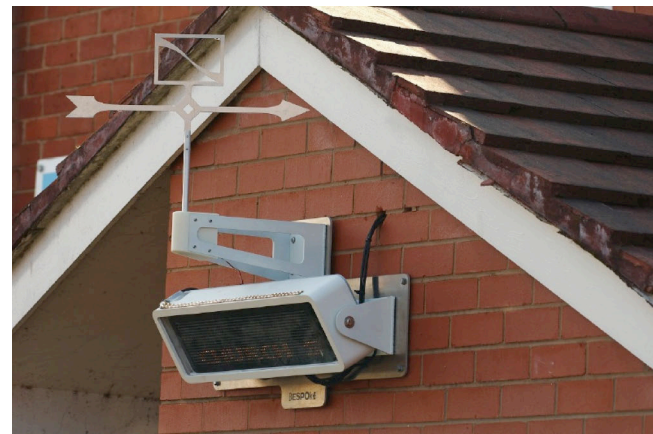
Figure 3. Wayfinder installed on a community housing office.
